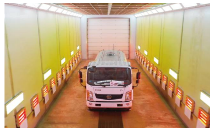
Baking integrated paint room
